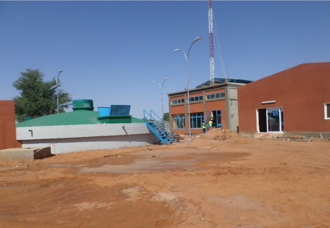
Treated water tank and other facilities
